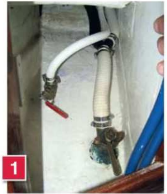
1 The Blakes seacock can be seen in the foreground. The junction with the black hose is where the holding tank and toilet outlets converge. Two hose clips are put on all connections, with tightening screws on opposite sides
